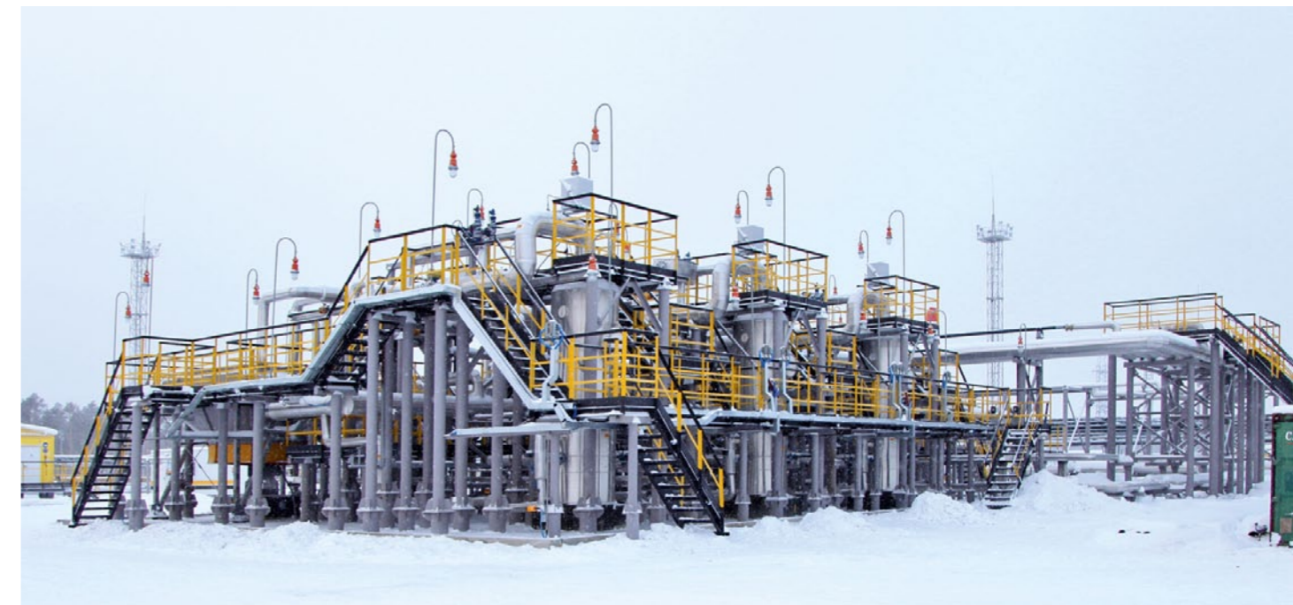
RN-Yuganskneftegaz has commissioned a new gas preparation plant to process the gas produced at the Ugut-Kinyaminskaya group of fields
