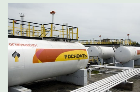
Thanks to the taken measures the operations of Rosneft subsidiaries during flood were in routine mode. On the photo: Khabarovsk tank farm of the RN-Vostoknefteprodukt
