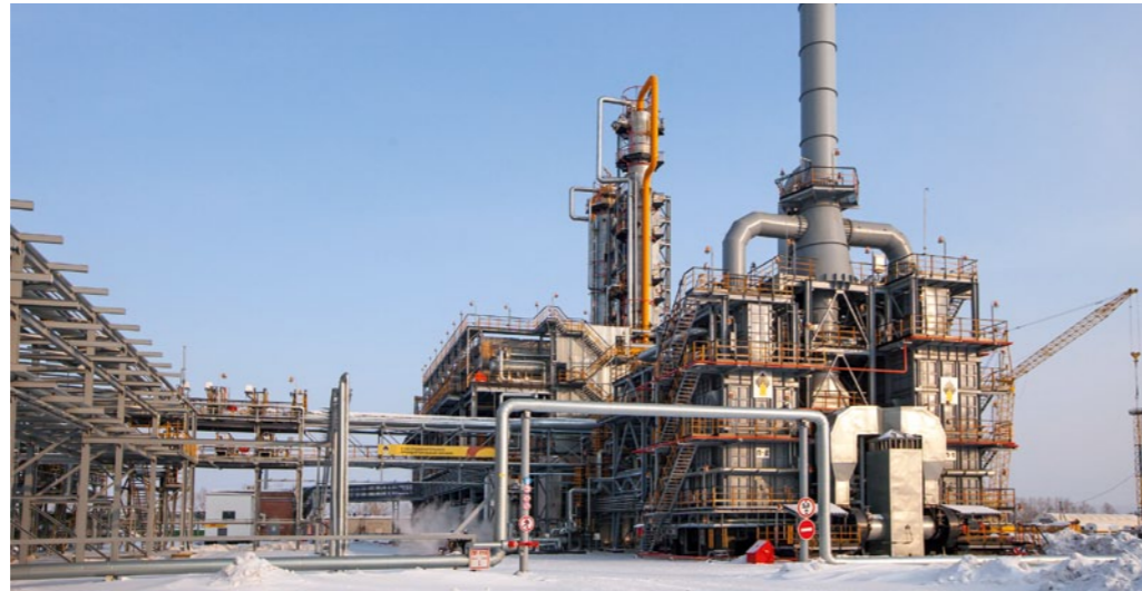
A major upgrade of the Komsomolsk Refinery is a project on the scale of the construction of a new plant. The program involves the construction of new hydrocracking, reforming, and coking units, and 25 other facilities
